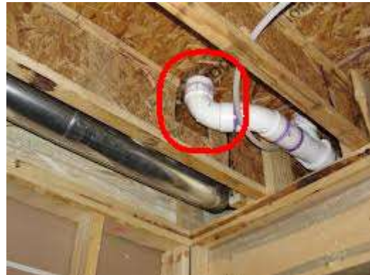
Figure 12-BIM enabled IPD should stop this kind of costly repair
